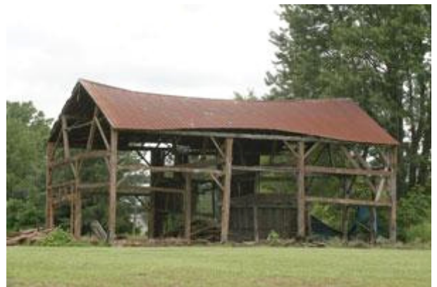
SPENCER TULIS/Finger Lakes Times An 1829 barn built and owned by village founder Samuel Bear on east River Street in Waterloo is being dismantled.
